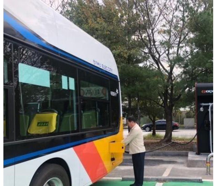
Figure 5: Fast charger for e-buses. Credit: Korea Electric Power Corporation (KEPCO).
